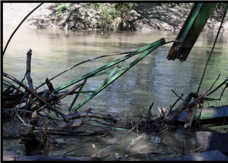
September 30, 2010 McIntyre Bridge rare wrought iron structural members are removed from a twisted mass of tree branches.
