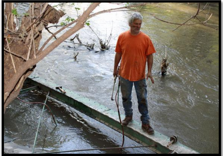
September 27, 2010 Nels Raynor (BACH Ornamental & Structural Steel from Holt, Michigan) begins dismantling the top chord section of the McIntyre Bridge
