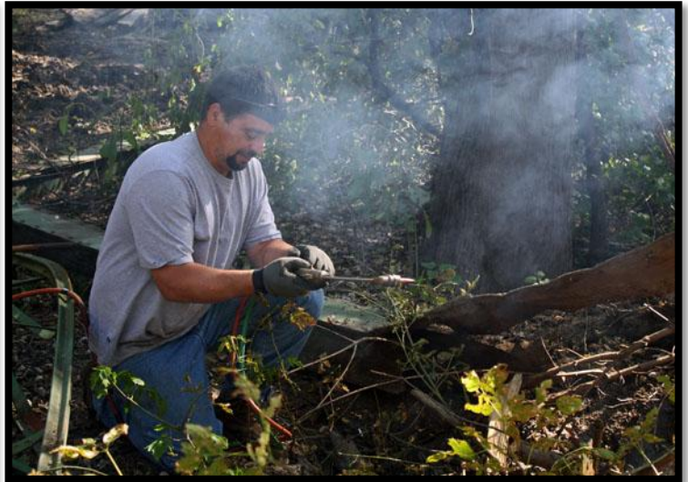
September 30, 2010 Shane Milliken (working with Nels Raynor) dismantles a top chord section of the McIntyre Bridge
