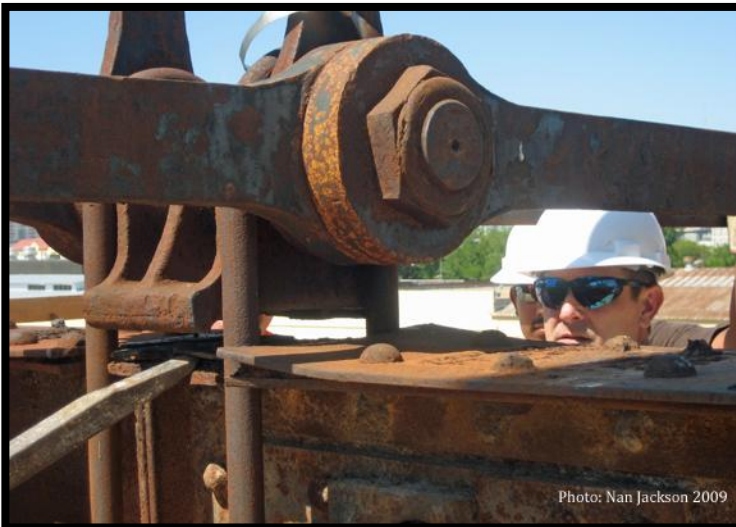
Riveted floor beam separated from a pin connection for inspection
