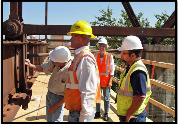
Patrick Sparks and Andrew Roberts inspects pack rust
