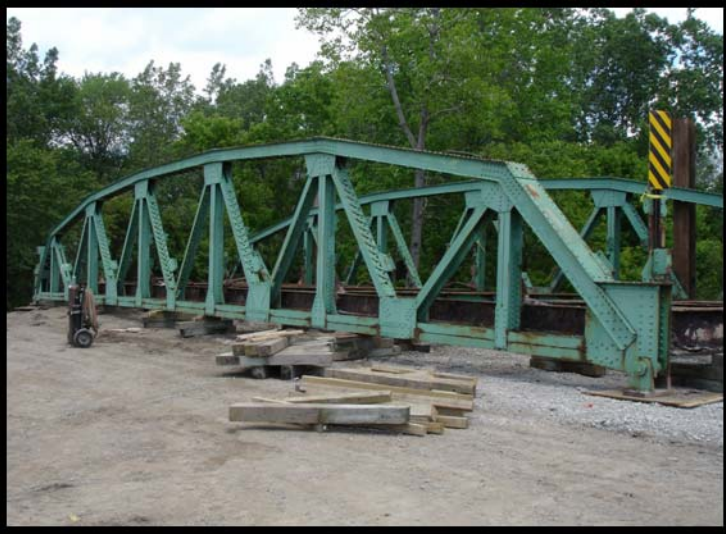
Bridge off the river and ready to dismantle in St Clair County
