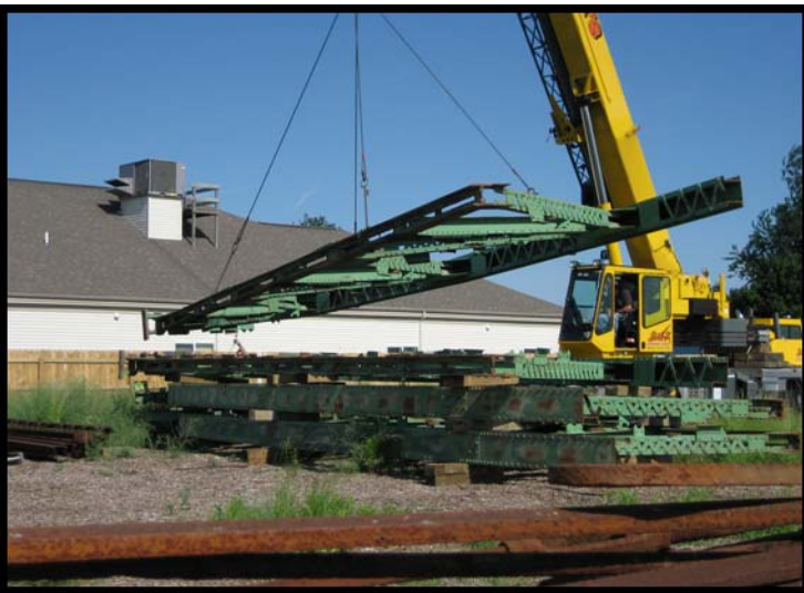
Buck from Buck's Crane positions the last half section of the Indian Trail Bridge
