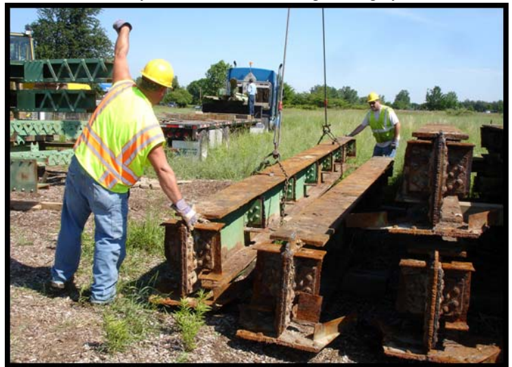
Calhoun County workers Mike and Steve unload the last Indian Trail Bridge member
