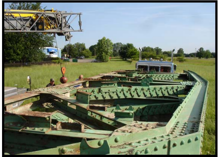
Safeway Trucking positions the Indian Trail Bridge truss sections at the Calhoun County Marshall historic bridge storage yard
