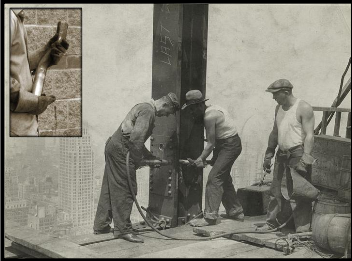
Rivet gang using rivet hammer (left) and holder-on "bucking bar" (right) in construction of the Empire State Building Photograph: Lewis Hine, 1931, NY Public Library Digital Gallery [Insert: detail of bucking bar of similar type]
