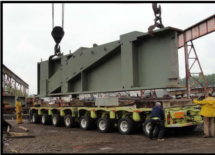
Loading 75-ton section of WTC Transportation Hub at Harris Steel, on a trailer with 64 wheels
