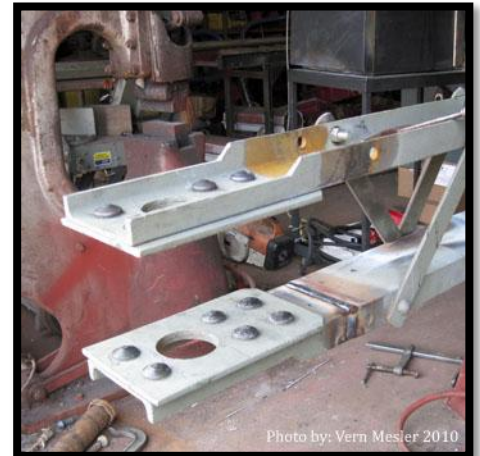
Replicated vertical pin connections are arc welded with full penetration welds to the original vertical channel
