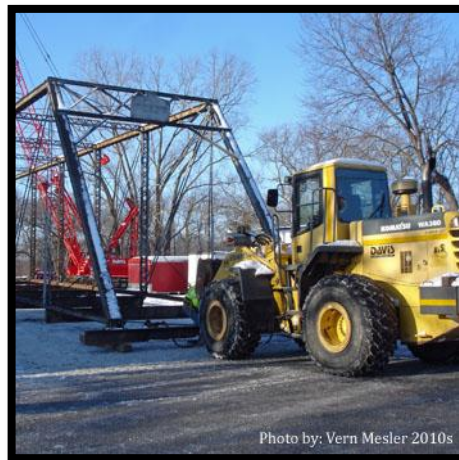
A span of the State Street Bridge moved through Bridgeport to its restoration area.
