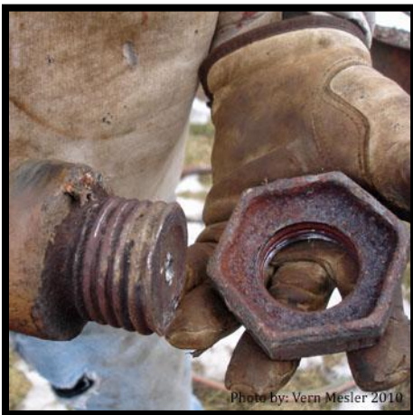
Nels Raynor holds a bridge pin and recessed nut removed from the State Street Bridge
