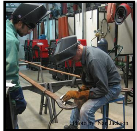
Photo by: Nan Jackson Vern Mesler pad welds section loss on an early twentieth century eyebar head with the SMAW process.
