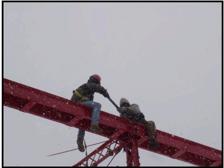
Wayne Conklin and Rob Denniston tighten a top chord bridge pin during one of the coldest days in January.
