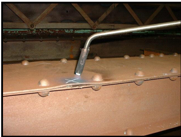
Heating pack rust buckle
