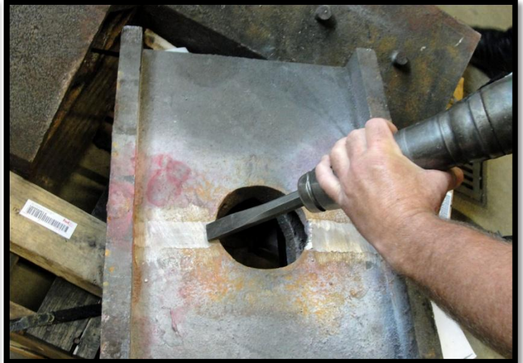
Joint preparation for braze welding begins with chipping using a pneumatic hammer to produce a joint that has a good anchor pattern. (Photo shows a previous repair.)
